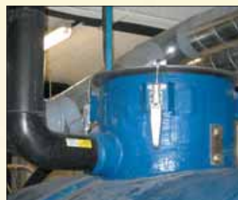
Tank inspection hatch showing the 110mm Geberit exhaust air pipe
