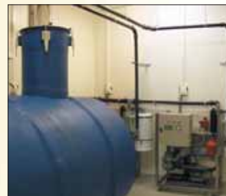
MV-5000/2-S storage tank with 2 x MV-7.5 vacuum pump modules
