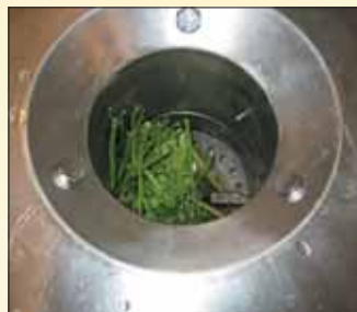
View of waste inlet with water flushing nozzles
