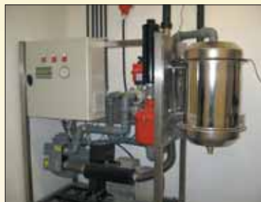
MV-7.5 vacuum pump and PLC control module
