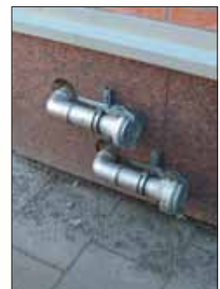
Emptying valve located to the exterior of the building
